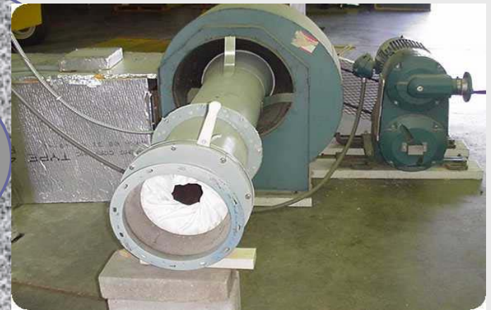
Inlet of 18 kW Heater
