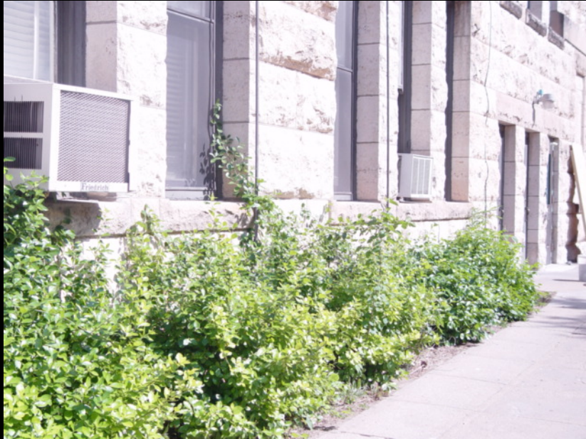
Shrubs too close to building
