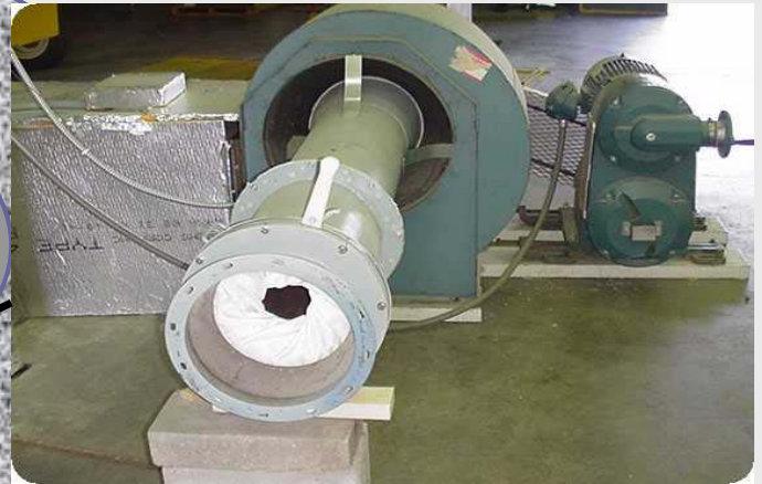
Inlet of 18 kW Heater
