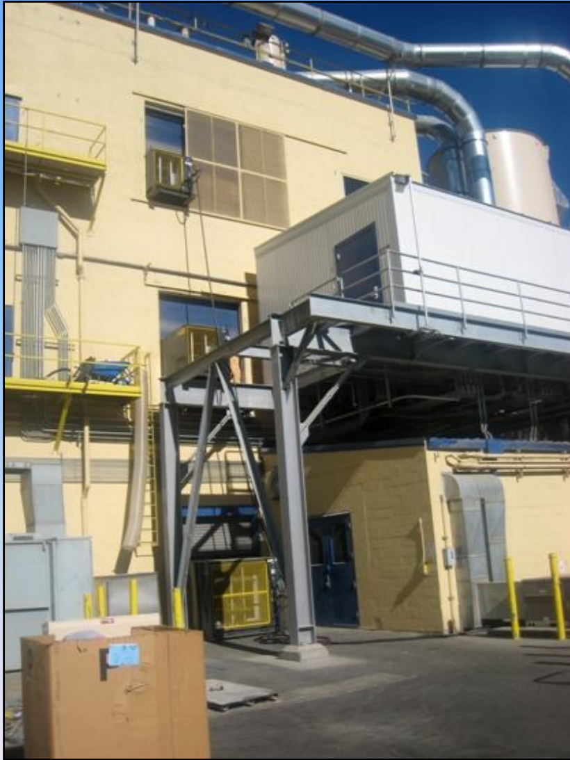
Heater Placement on multiple floors
