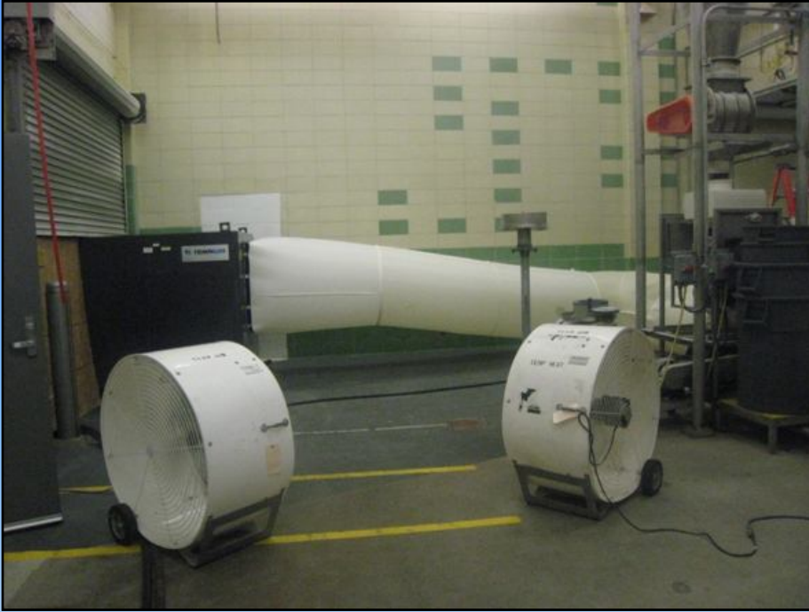
Heater Partially inside Packaging Plant
